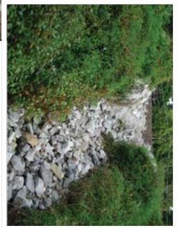
2) Temporary Repair of Damaged Stormwater Infrastructure
