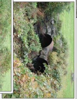
4) Invasive Plant Growth Interfering with Stormwater Drainage/Choking Wetland System
